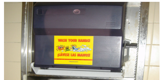
Removed accessible tri-fold dispenser w/ inaccessible fixture
